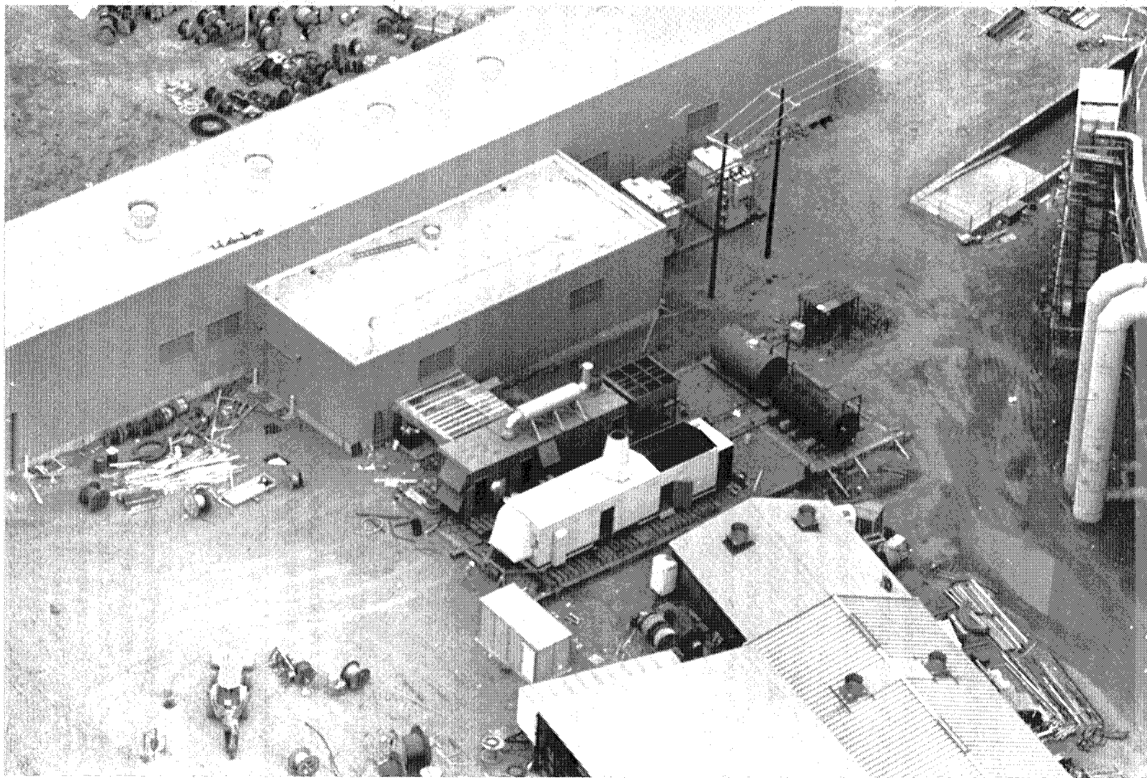
Photo 3-3. Gray and White Backup Diesels
